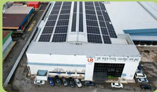
URC Malaysia's solar roofing project reduced energy consumption by 448,812 MJ.
