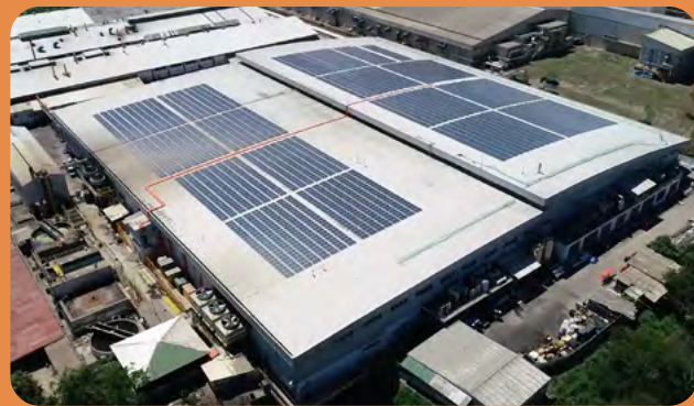
Solar panel-equipped URC plants completed in 2025 are projected to save PHP 24 million in annual cost savings.
